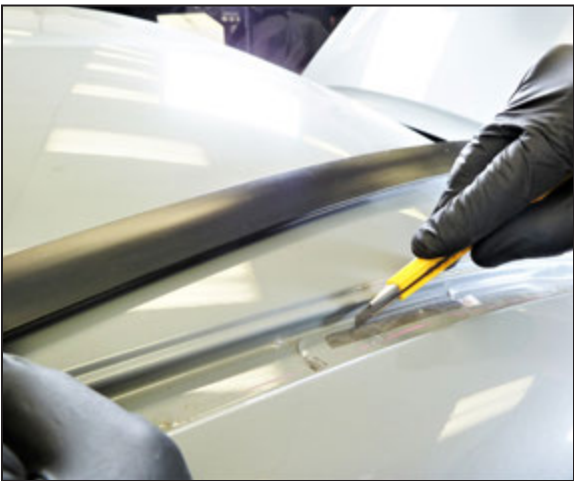
17. Using a knife, slice the sealing tape to allow access to the inserted nuts. NOTE: Do not remove the tape, slicing the tape will allow the bolt to pass through.
