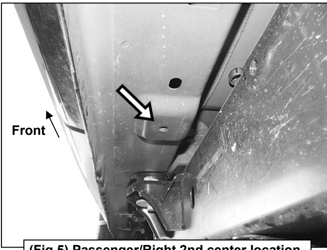
(Fig 5) Passenger/Right 2nd center location
