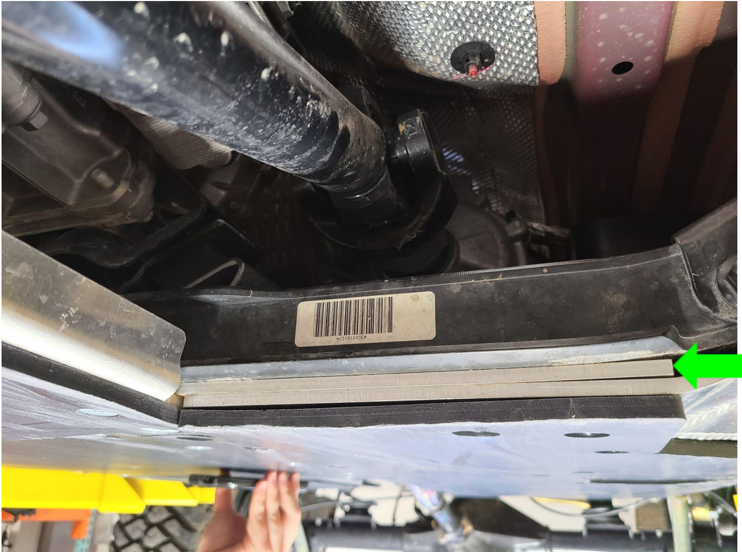
Figure 9: Aluminum Spacer (Figure 3 Item #8) shown with green arrow and sandwiched in between the fuel tank, transfer case, engine skid and the frame
